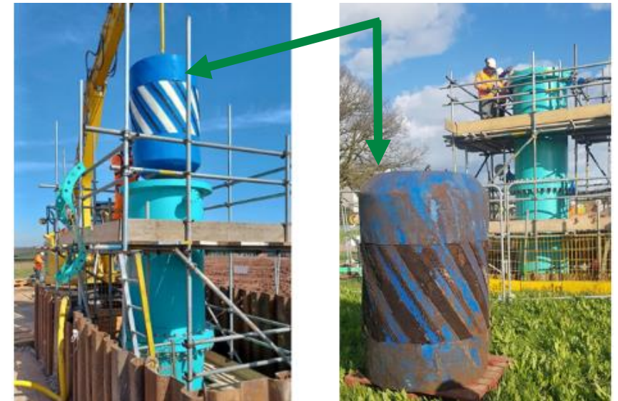
Before and after the cleaning of the Vyrnwy aqueduct using our 'pigs'!
