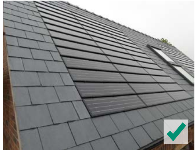
Figure 105: Integrated solar panels on slate roof.
